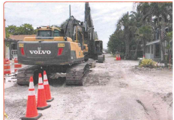
The contractor working to install the gravity sewer eastward down 11th Street South.
